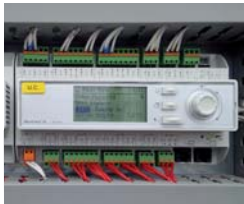
Controller box upgrade
